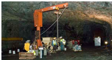
Figure 6: CAI supervisor Jim Norris and Ramiro Hernandez of Shotcrete Technology inspect batch plant in Transition Cavern. The jib crane was recycled from Homestake's wash rack at the surface level
