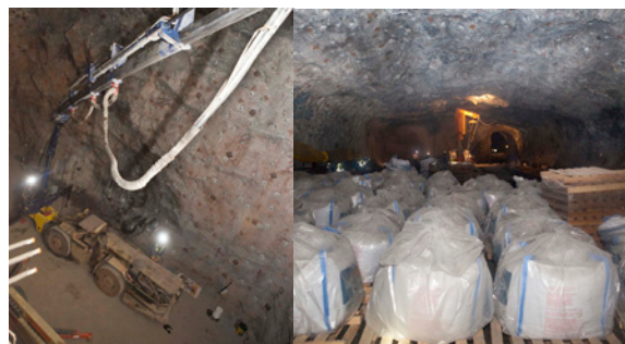
Figure 10: (left) Robotic arm in Davis cavern can be operated from the ground to apply shotcrete in hard-to-reach places; (right) Bags of shotcrete with hoist in background
