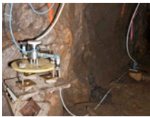
Figure 4: Wall mounted Budker style tiltmeter (foreground); Pedestal mounted Tevatron style tiltmeter (background)
