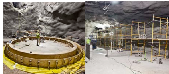
Figure 7: (Left) Circular wooden form surrounds concrete ring which will hold the water tank used to protect the LUX dark-matter detector in Davis Cavern; (Right) Masons have laid 20 to 25 percent of the concrete-block walls at the Davis campus
