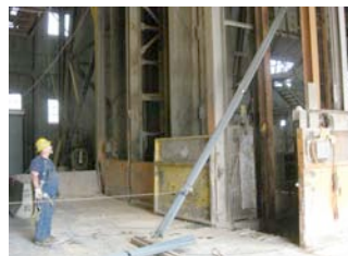
Figure 5: Infrastructure Tech Danny James lowers a bundle of rebar down the Yates shaft
