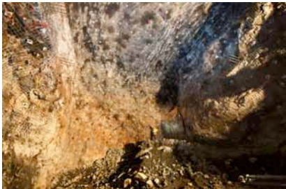
Figure 1: Undergruond Construction Project Engineer Wendy Zawada (in yellow jacket) in large Davis Cavern
