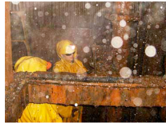
Figure 3: Infrastructure techs cut old pipe out of the Ross Shaft under wet conditions
