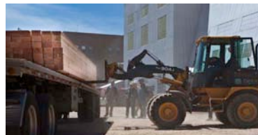
Figure 10: Infrastructure Tech Kevin Ehnes operates the loader as new shaft guides are installed at the Yates Shaft to provide better access to the 4850 Level
