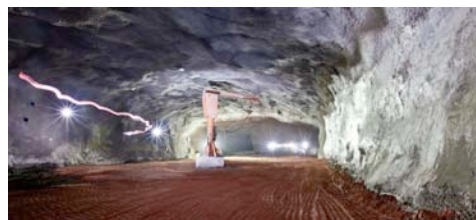
Figure 12: Shotcreted walls and ceiling in Transition Cavern with engineered fill on the floor
