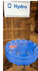
Figure 7: Several members of the installation crew autographed the top cap of the deep-water pump column
