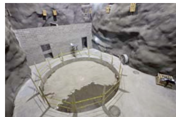
Figure 11: Davis Cavern viewed from south end, from tunnel leading to Transition Cavern. The circular water tank will support the water tank for the LUX dark-matter detector
